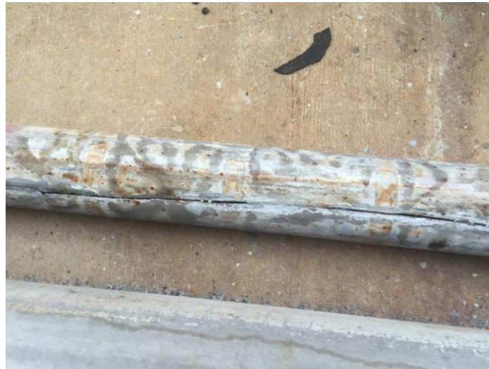
Figure 5: Water washing system cracking due to corrosion.
