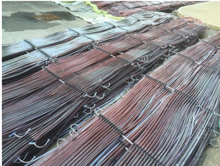
Figure 10: Discolouration of the PFA tubes due to fly ash contamination.
